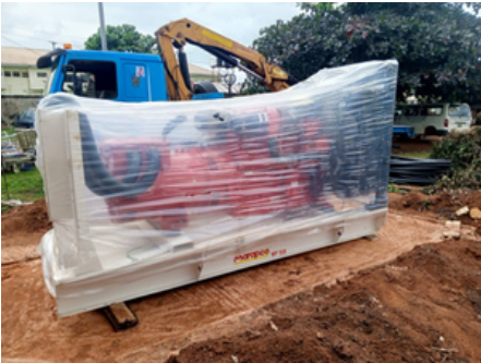
500 kva power backup generator delivered to ISTH in Irrua, Nigeria
