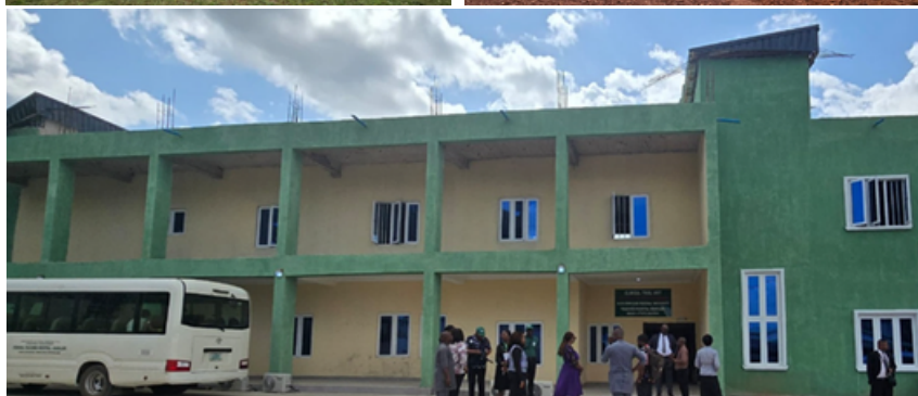
Progression of construction from grass area to a 2-story main CTU building at AEFUTHA, Abakaliki, Nigeria
